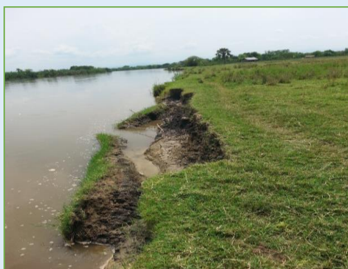
Degraded /collapsing Semiliki riverbanks
