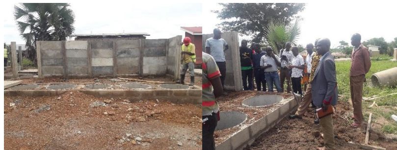
Construction of the super structure in Alukot Primary School in Oyam District
